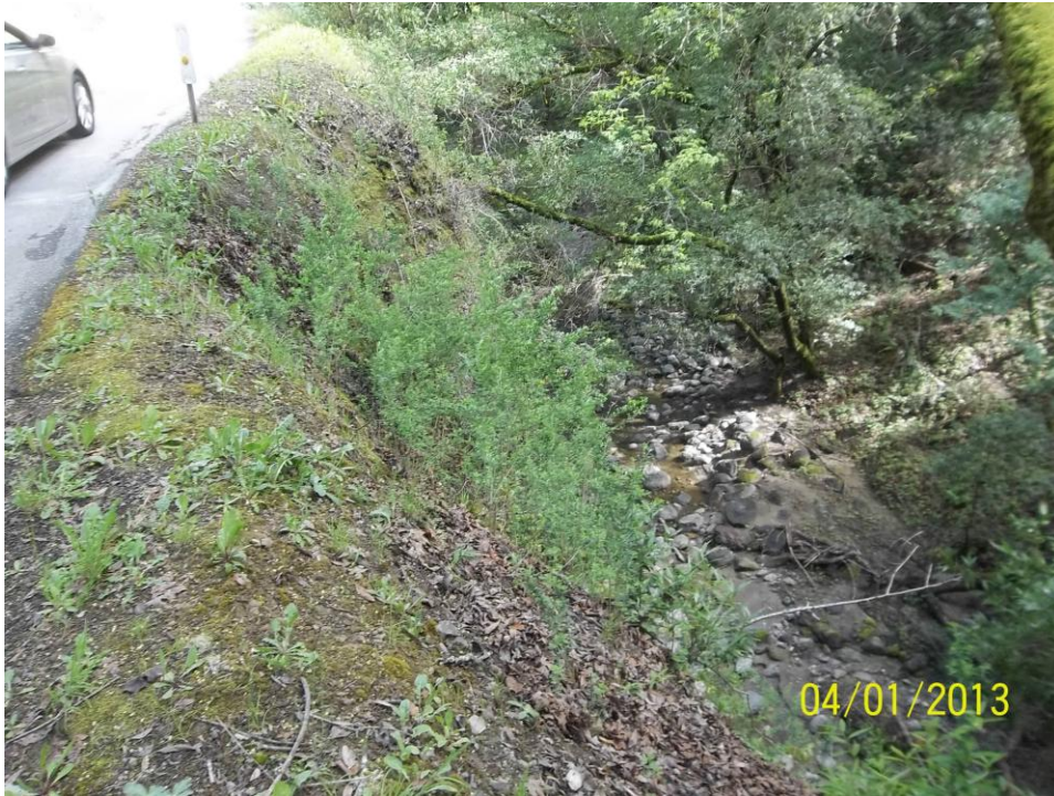
Photo 5 – Site 2: Photo showing the smaller slip-out immediately north of the slip-out shown in Photo 6. Note the colonization of invasive French broom in the disturbed slide area.
