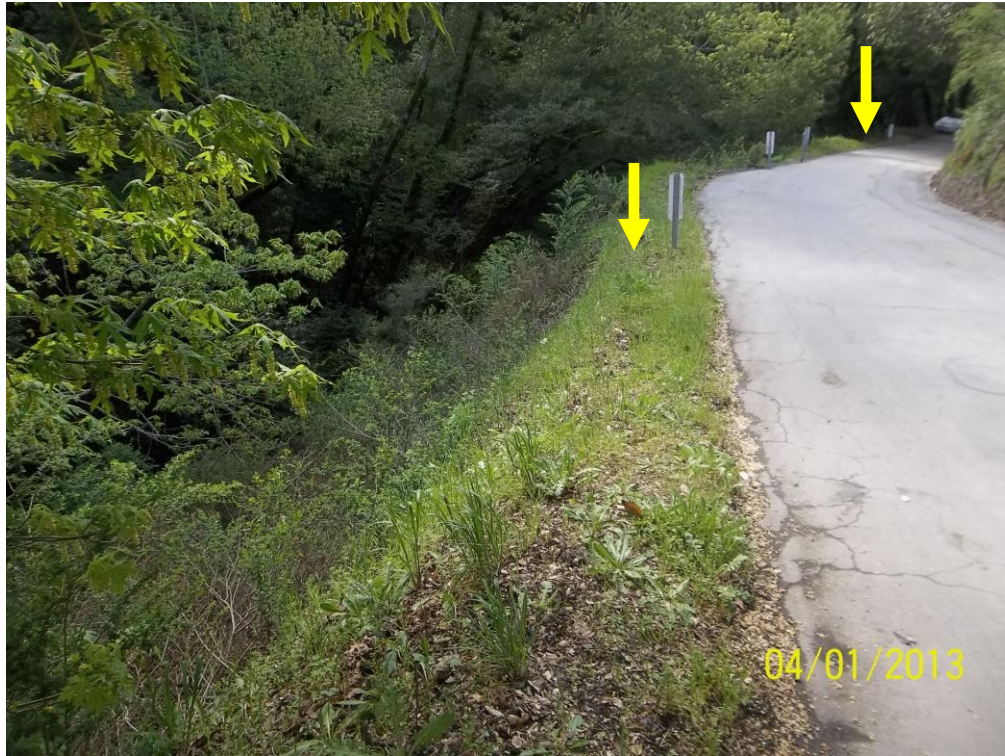
Photo 4 – Site 2: Photo looking north at the adjacent Site 2 slip-outs, located along Alpine Road approximately 250- to 350-feet from the Joaquin Road intersection.
