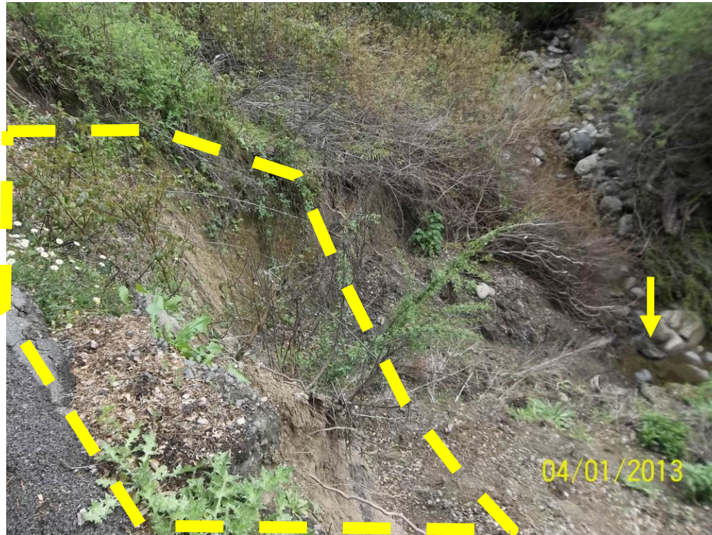
Photo 2 – Site 1: Photo taken on April 1, 2013, following additional bank failure due to large storm events in December 2012. The slip-out currently extends from the roadway to Corte Madera Creek. The County proposes to remediate the upper portion of the embankment (area indicated by dashed line). Location of Corte Madera Creek below the slip-out is indicated by arrow. The creek was dry during a site visit on July 26, 2013.
