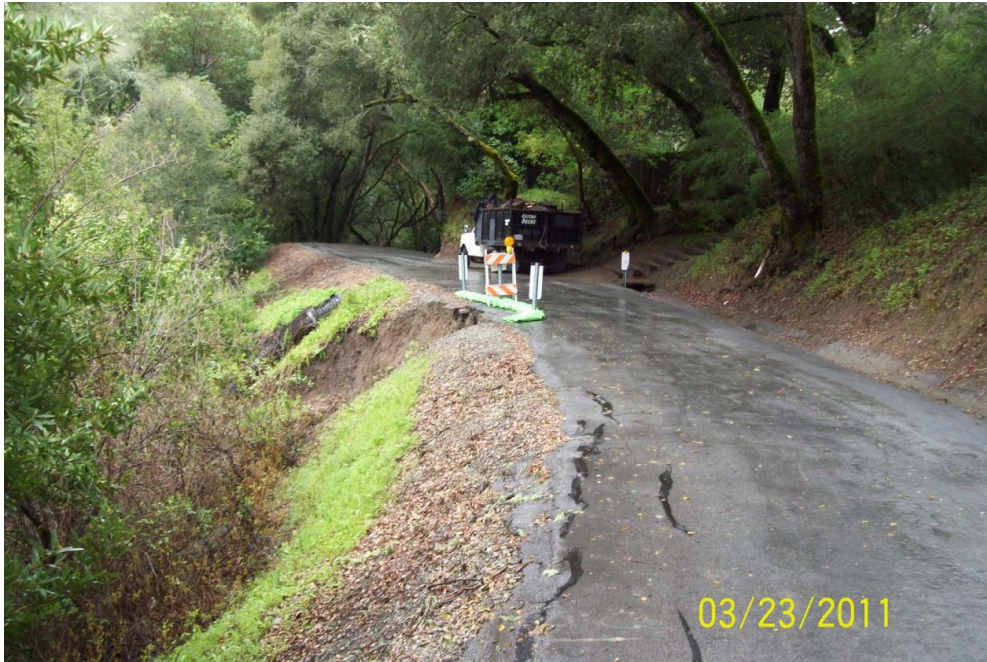
Photo 1 – Site 1: Photo taken on March 23, 2011, shortly after the slip-out was first detected. The slip-out resulted in a near vertical drop from the edge of pavement down to approximately 25-feet below the roadway surface.
