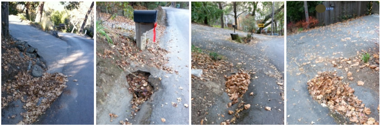
Examples of clogged driveway pipes throughout our neighborhood
